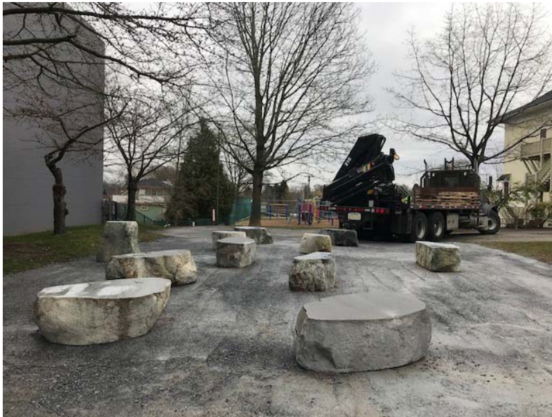
Installation might occur over a few weeks depending on the scope of the project.
